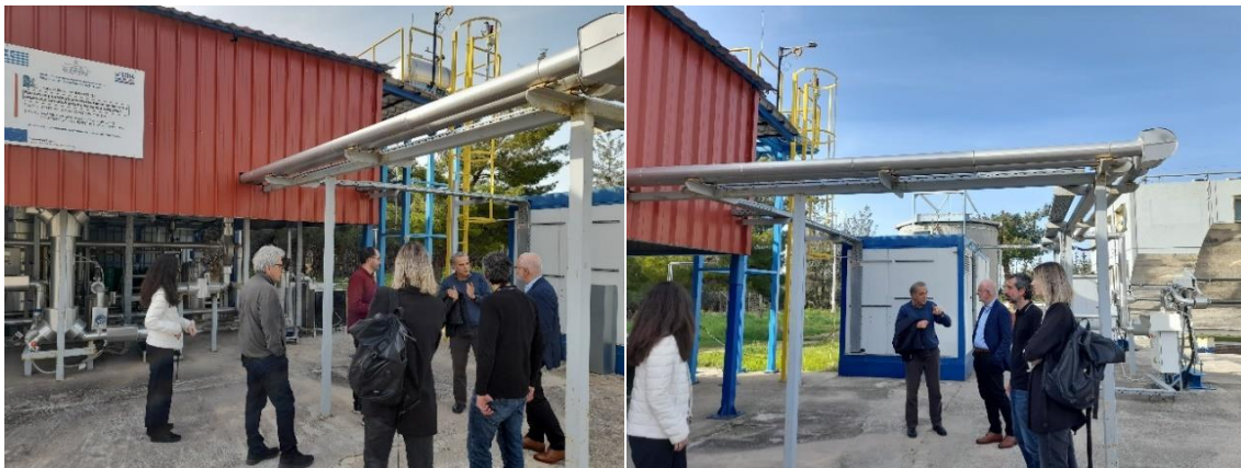
Figure 1. Tour at the concentrating solar thermal field and thermal storage infrastructure in March 2025
