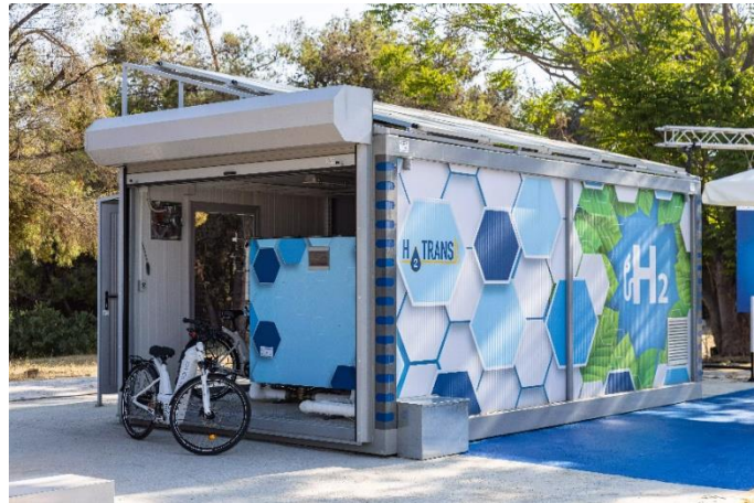
Figure 4. The prototype hydrogen thermal compressor installed at the NCSR campus combined with hydrogen production and storage units
